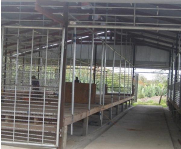
Plate 8 Raised slatted floor pens under construction with high roofing and adequate ventilation
